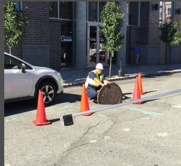
18 th Street Pump Station – W 18 th St.
