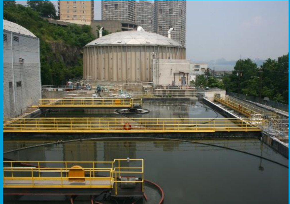
River Road Wastewater Treatment Plant 6400 Anthony M Defino Way, West New York 10 MGD
