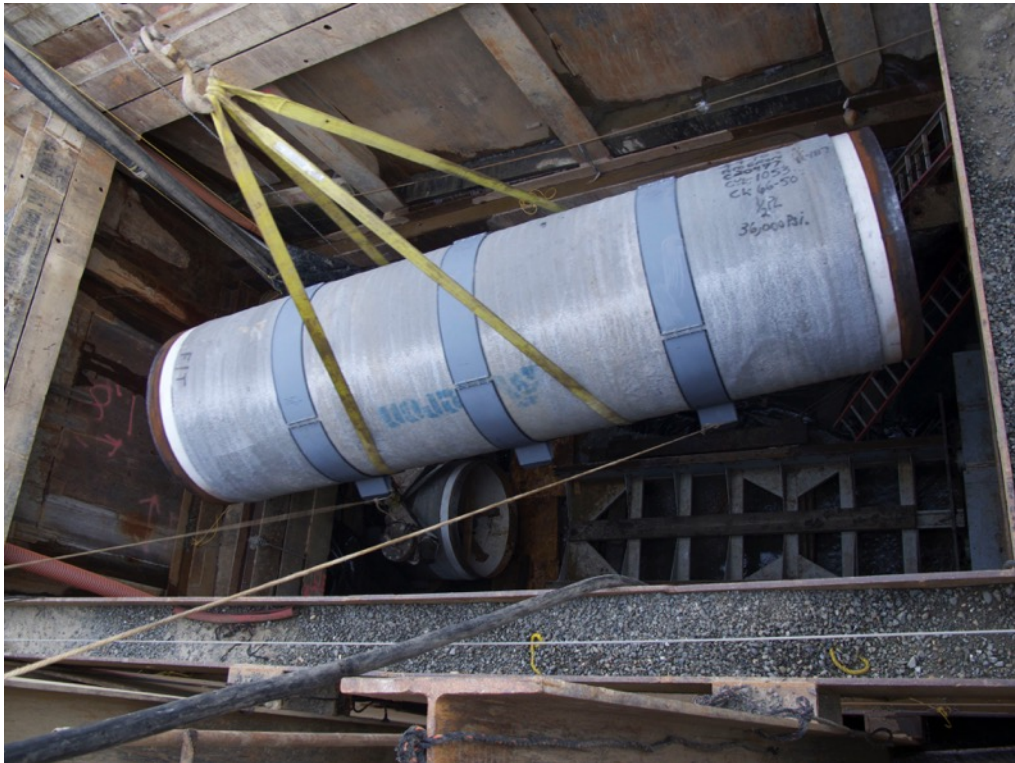
Siphon Alameda, CA
